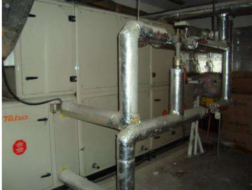
Bodrum kat – Klima Santrali
